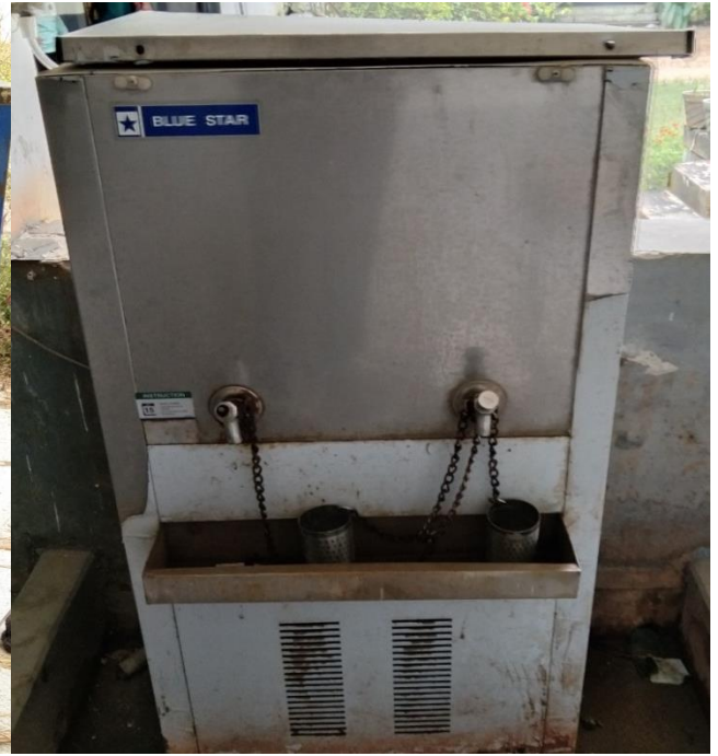
Fig. 18 Water purifier pump
