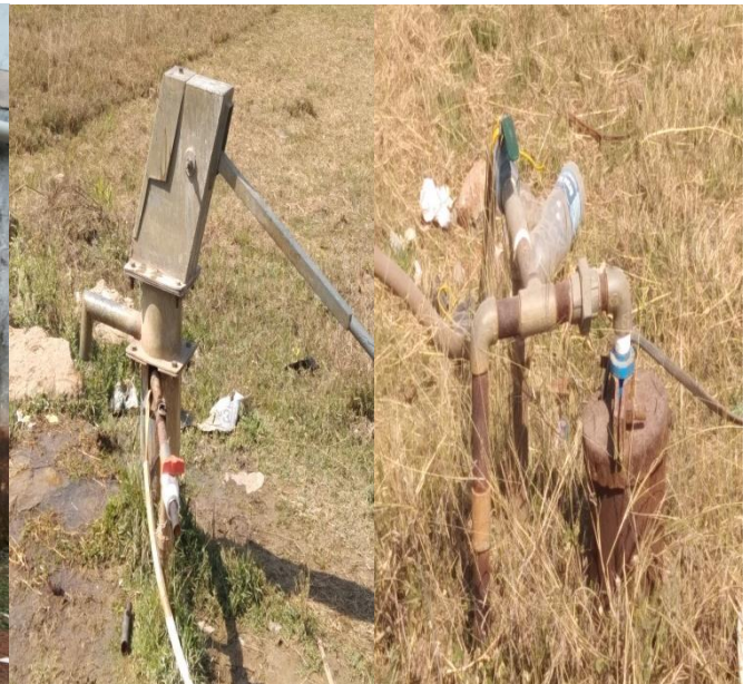
Fig. 20 Two pump set
