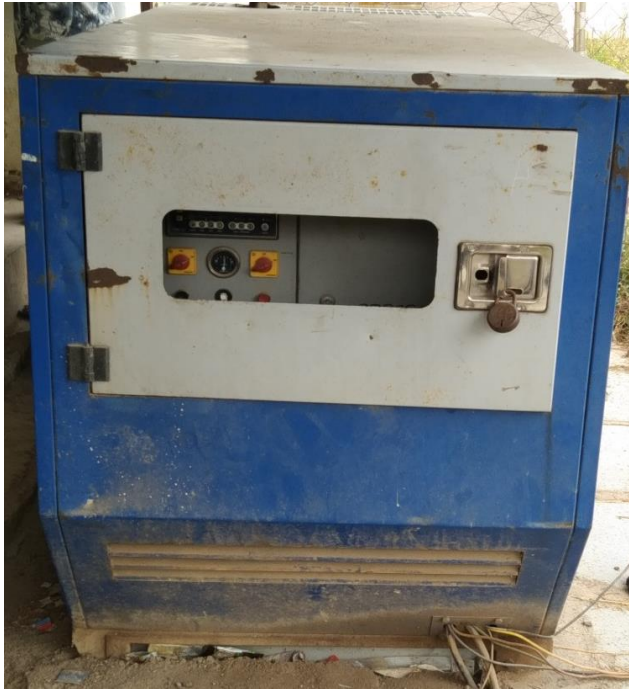
Fig. 17 Generator for Electricity
