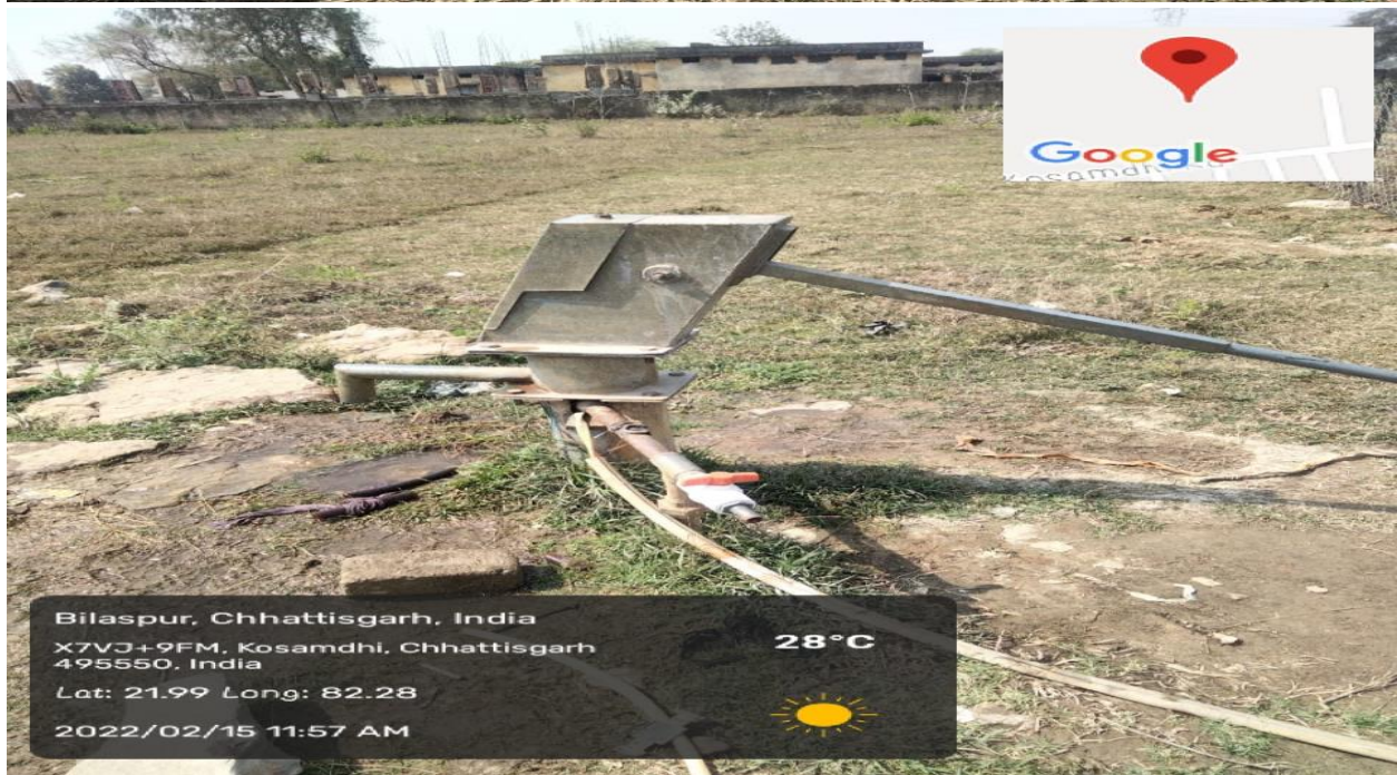
Water Pumps in front of Main Building and RUSA Building
